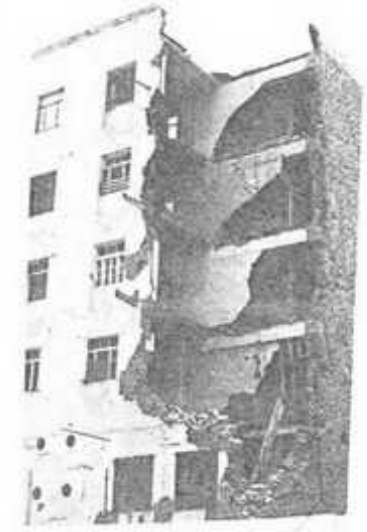
Plate 10 Clear View of Damage
